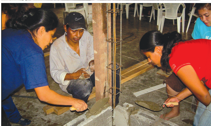
Top: RYS participants in a group-building exercise in Guyana, July 2005, Second: Foot-washing ceremony in Malaysia, June 2006, Third: Mixing concrete in Guatemala, July 2006 Bottom: Building a kitchen in Honduras, August 2007
