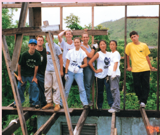
A divine demolition squad poses in the ruins of a house it is about to tear down
