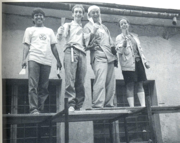
A moment's pause from scraping the army barracks which would be transformed into a kindergarten building.
