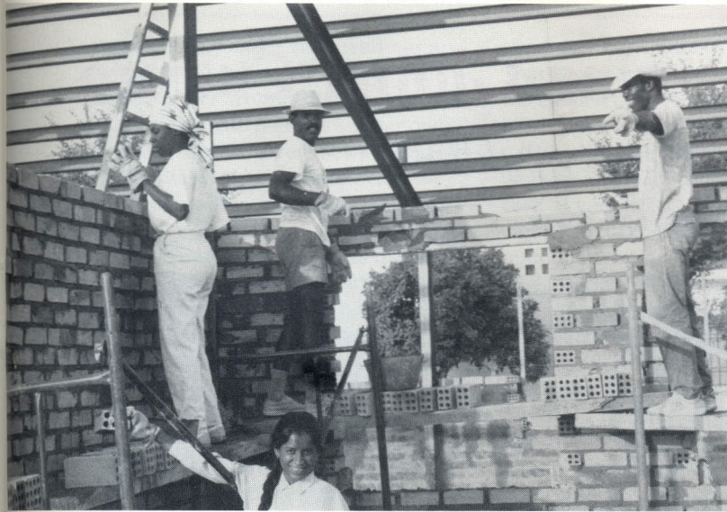
The Sevilla group became proficient bricklayers in the process of building their day-care center.
