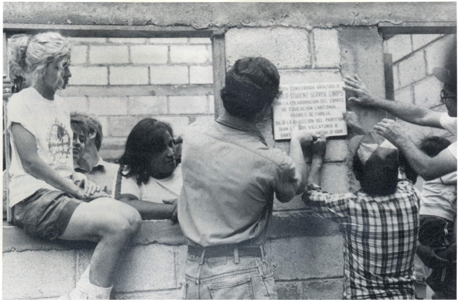
Setting the commemoration plaque at the completion of the school construction project.
