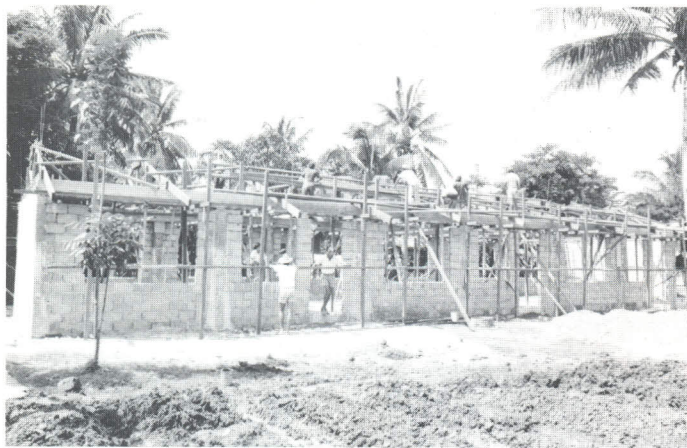
School construction in progress in Iloilo. This building will house three elementary classrooms.
